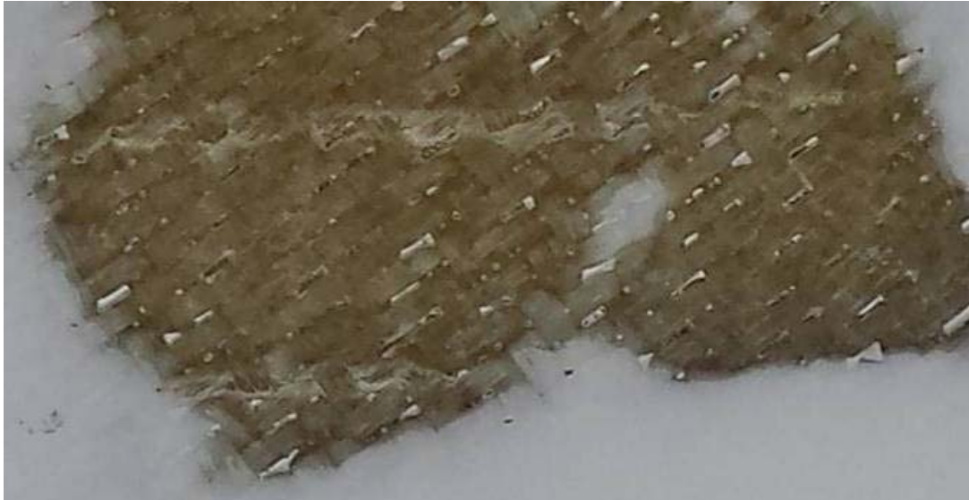
Figure 2. A crack area after gelcoat removal over glass FRP
